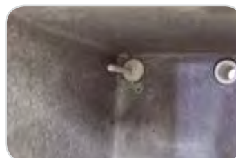
Thermocouple and ventilation chimney in the furnace chamber
