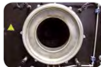
Retort of PKRC furnace
